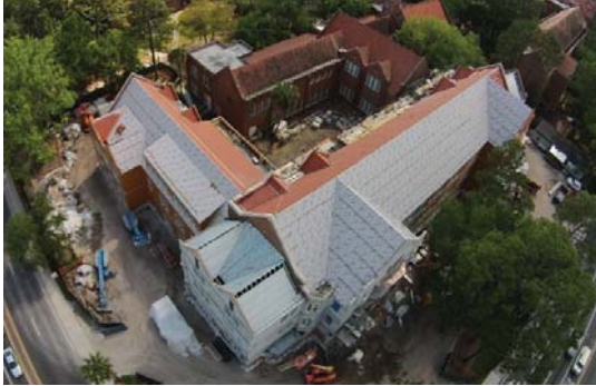
Figure 1 Overall construction progress image as of August 2014 captured via an unmanned aircraft
