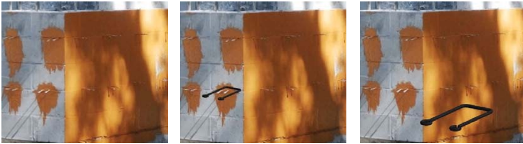
Figure 7 Copper flashing noted in video of brick veneer installation process
