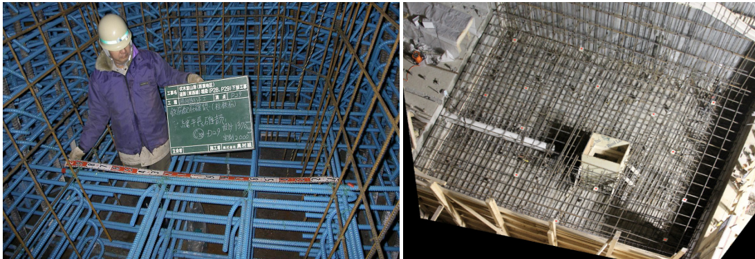
Fig. 1: a) An inspector measuring rebar spacings (Golparvar-Fard et al. 2010); and b) the safety hazard created through the density of the rebar layers for the inspector
