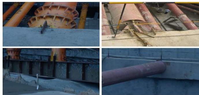
Figure 6: The noncompliant steel support (partial)
