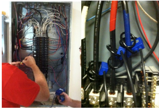
Figure 1. Installations of Power Meters
