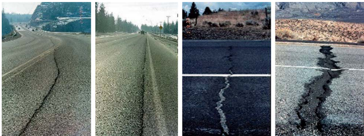
Fig. 66.3 Top two retrieved images using the “longitudinal crack” and “transverse crack” keywords (further annotated with “non-fatigue crack”)
