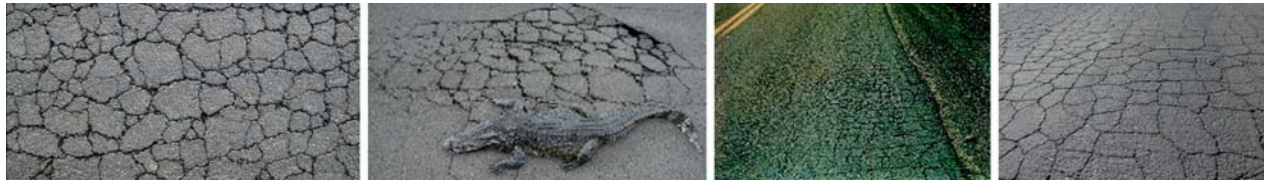
Fig. 66.4 Top two retrieved images using the “alligator crack” and “fatigue crack” keywords (further annotated with “fatigue crack”)
